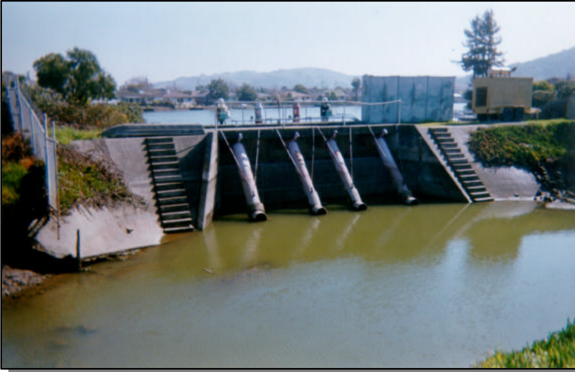
Pump Station at Lagoon No. 1.
