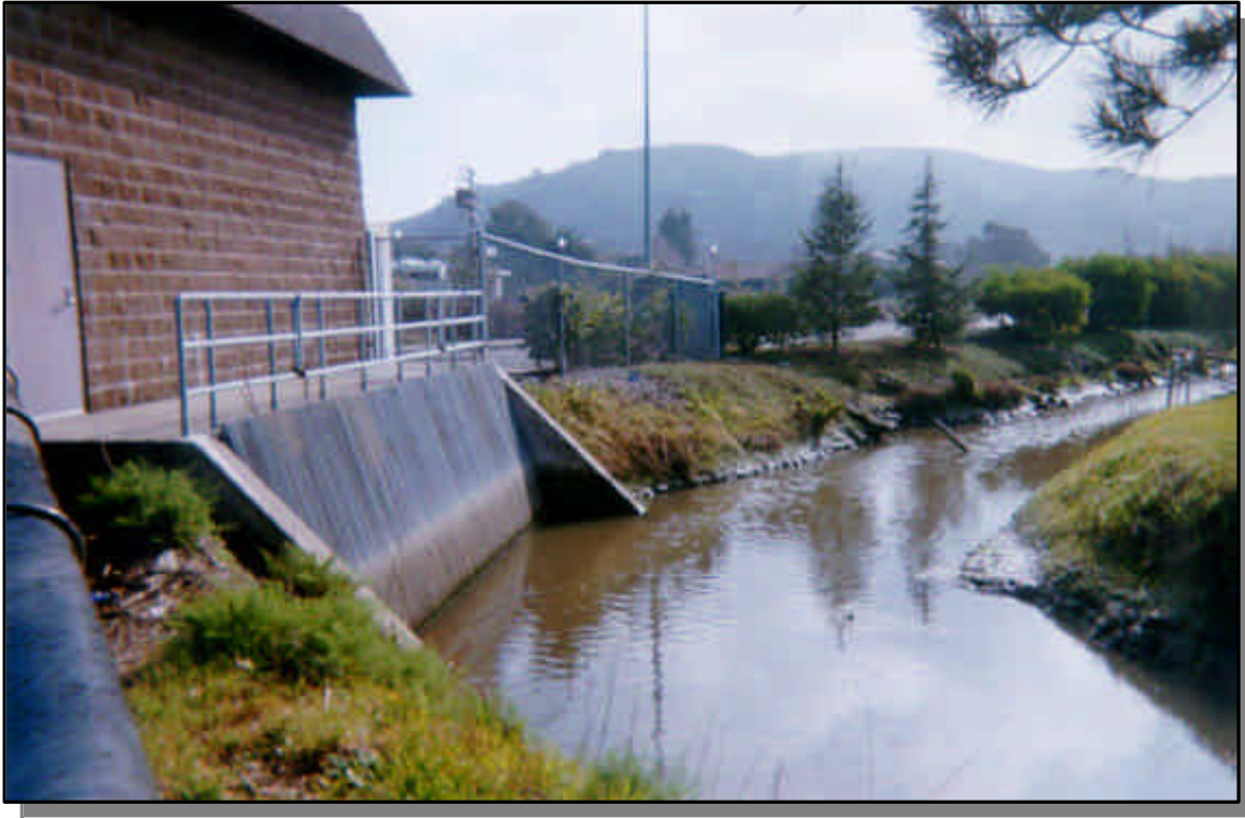
Pump Station at San Clemente Creek.
